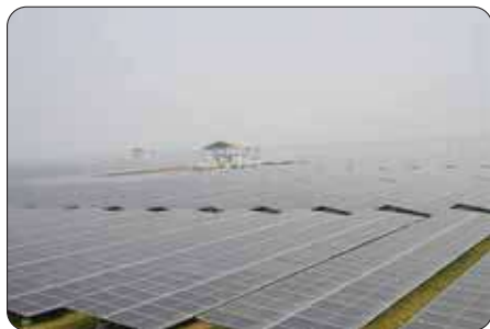
Figure: 200 MW Teesta Solar Park, Gaibandha
