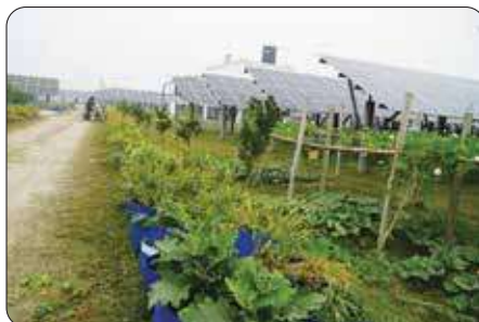
Figure: 30 MW Intraco Solar Park, Lalmonirhat
