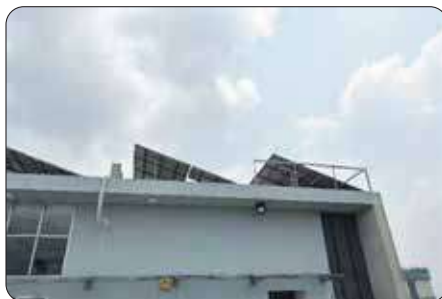
Figure: Net Metering Rooftop Solar
